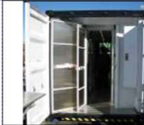
7 Racks plus Network
